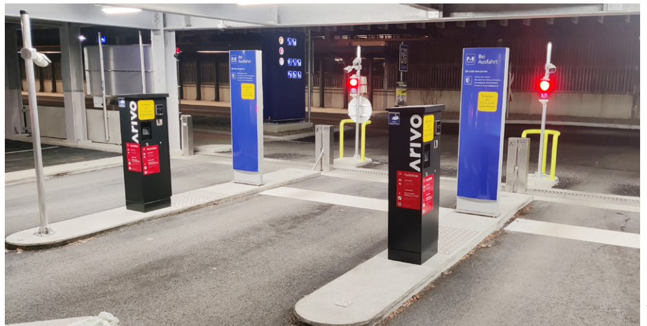
With Arivo's parking monitoring system, only commuters who actually use Park & Ride facilities can park there.
