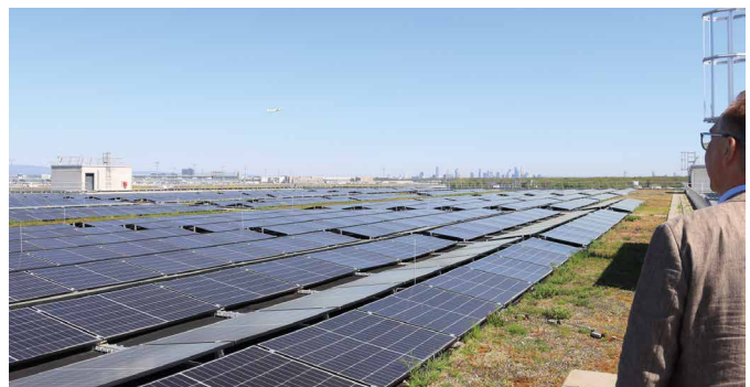
Gerald Krebs looks out over the photovoltaic system on the roof of the car park. This can supply the electricity needs of around 900 households.
