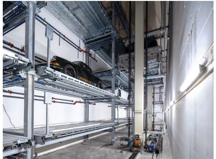
The WÖHR Multiparker 740 stacks 28 vehicles across four levels.
